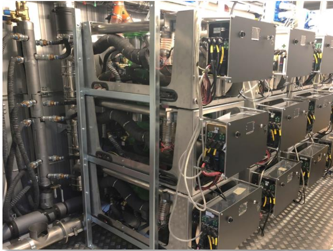
Enclosed set frame is for 3 stacked engine units.
